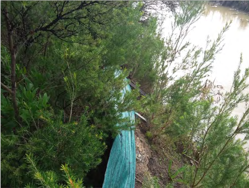
Silt fencing between habitat buffers and swales needs to be removed
