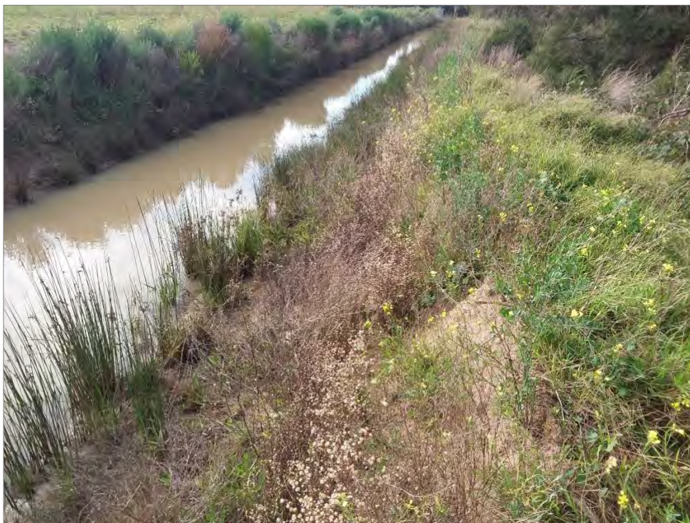
Dumped fill between the north-south habitat buffer and abutting swale
