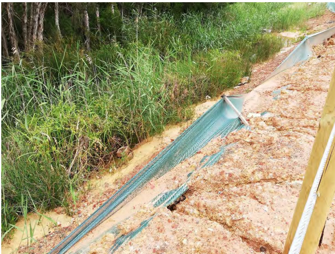
Sediment fencing has collapsed, with erosion channels running beneath the fencing, along the northern edge of the swale in the west of the site. Sedimentation of the water can be seen.
