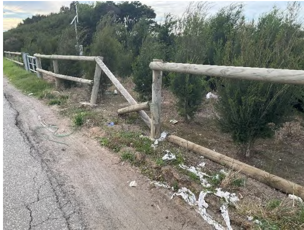
Photo 23. Damaged northern perimeter fencing
