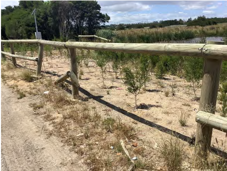
Photos 24. Damaged perimeter fencing next to the entryway at the northern boundary.
