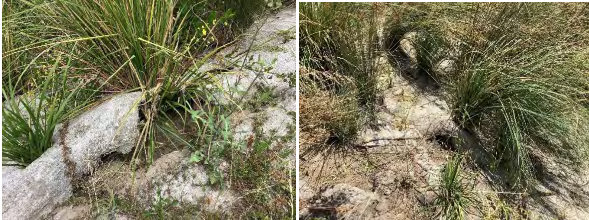
Photo 11 & 12. Representative unpinning of matting caused by plants outgrowing the holes
