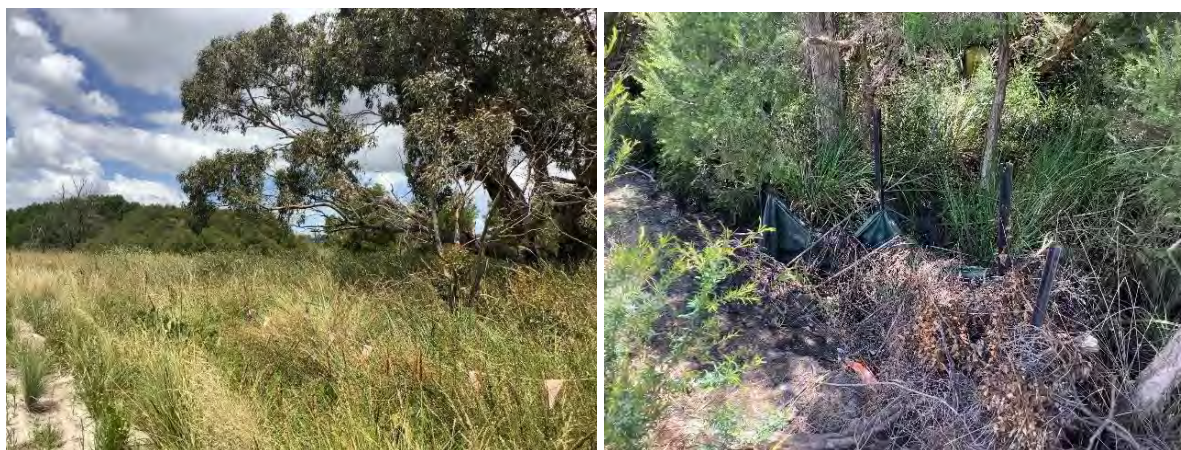
Photo 30-31. Rope bunting along the southern portion of the revegetation track (left) and broken sediment fencing (right).
