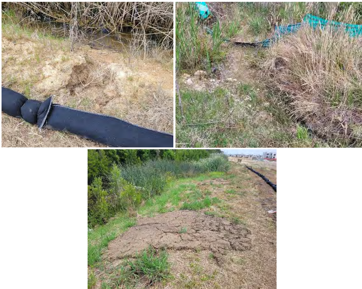
Photo 3. Photos of the soil erosion and disturbance mapped in the project site.
