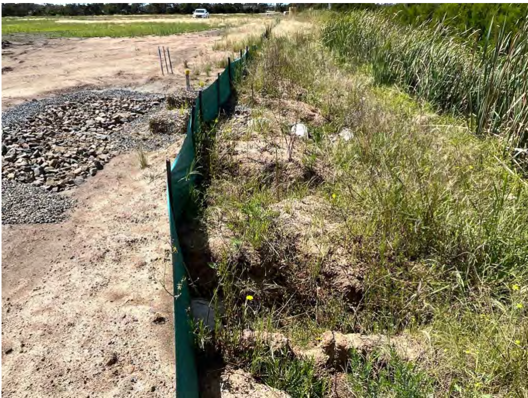
Sediment fencing in good condition, with efforts to control erosion through the use of rock fill, hay bales and sandbags along the northern edge of the swale in the central part of the study area.
