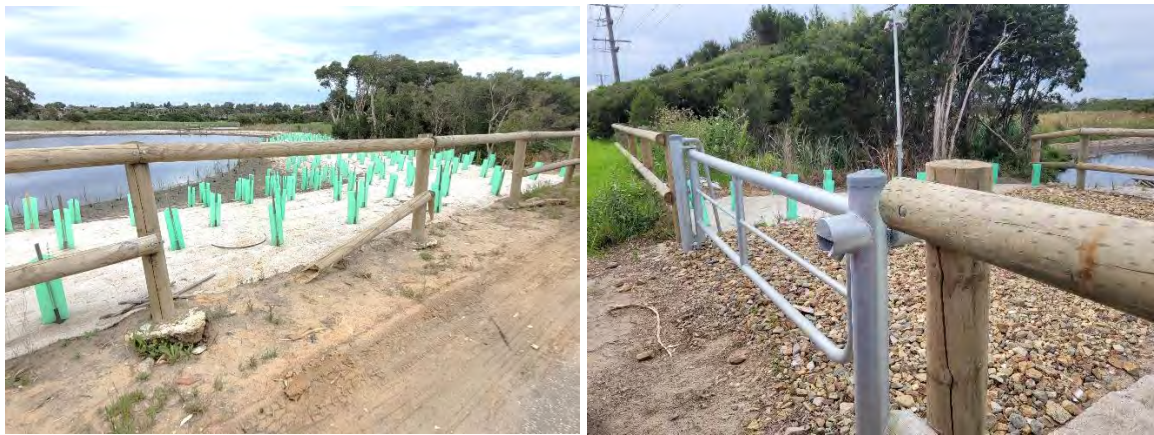
Photos 17-18. Damaged perimeter fencing and the entryway at the northern boundary.
