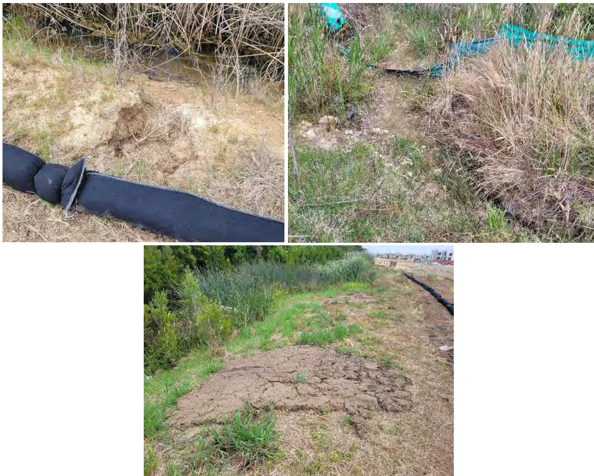
Photo 3. Photos of the soil erosion and disturbance mapped in the project site.
