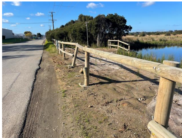
Photos 15. Damaged perimeter fencing next to the entryway at the northern boundary.
