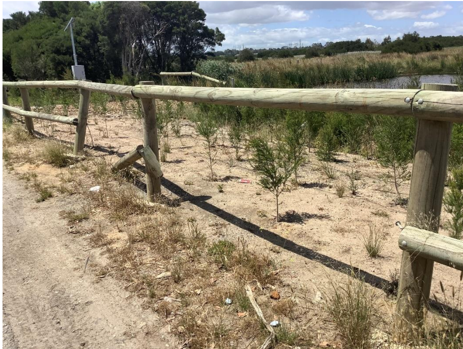
Photos 24. Damaged perimeter fencing next to the entryway at the northern boundary.
